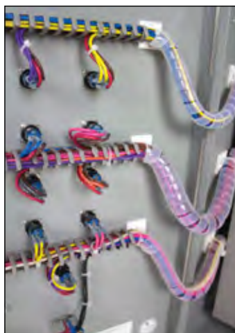
Door Device Terminations
