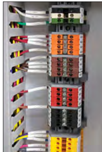
Labeled Terminal Blocks and Wires
