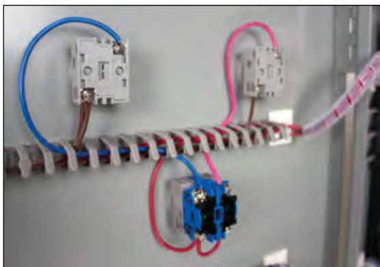
Door Device Terminations
